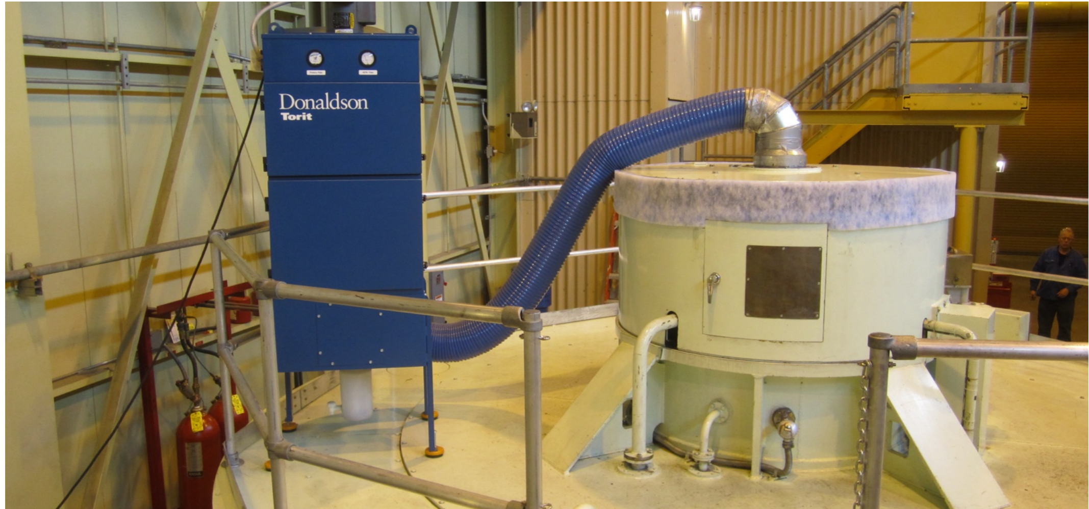
Donaldson Torit Mini-Mist Collector used in power generation application.
